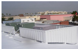
Metal Roof Equipment
